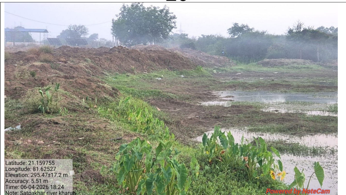
View of Desilting/overburden removal at the right bank of river Kharun by WRD (Towards Datrenga village side), Dist-Raipur
